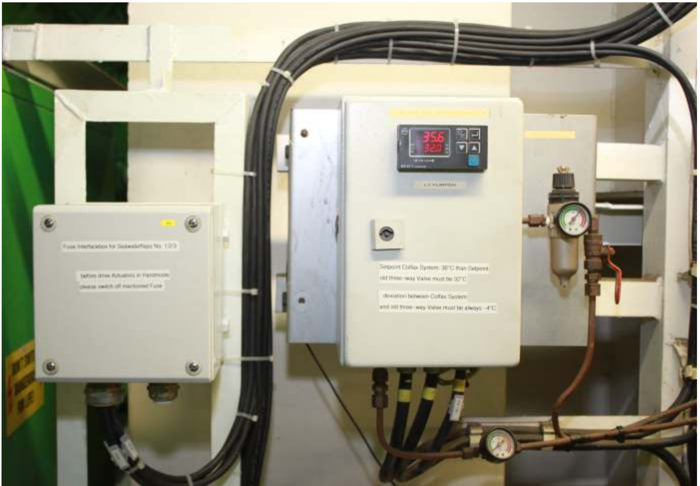
Wiring box (left) for the sensors of the CM-1000 system. Control box (right) for the controller drive of the three-way valve in the original controller of the LT cooling water system. On the Kyoto Express, its set point is always 4 °C below the set point of the CM-1000. This ensures that the "old" and "new" controllers do not mutually influence each other.
