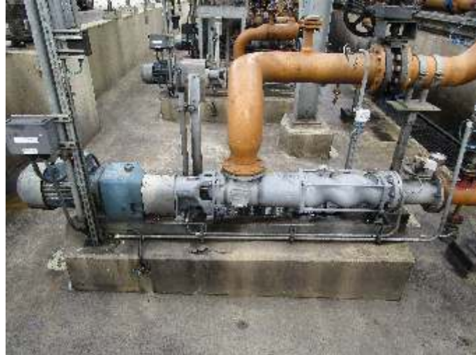
Progressing cavity pump in the main used oil unloading station.
