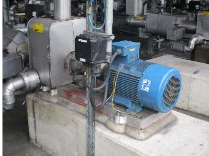
Centrifugal pump providing column circulation (liquid: base oil)
