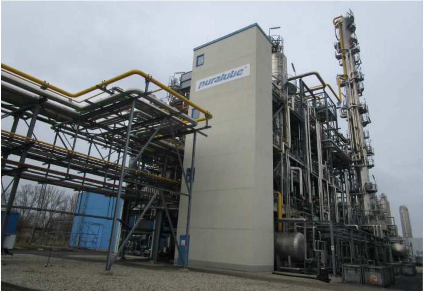
Process plant HyLube2
