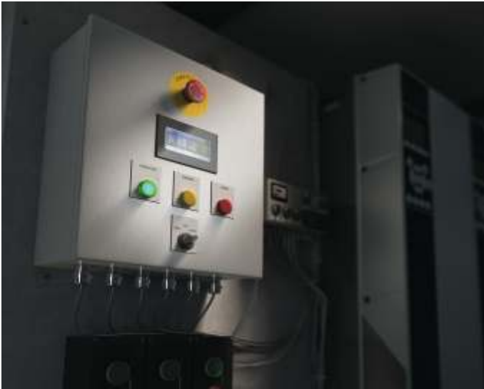
CM-1000 intelligent controller installed in engine room.
